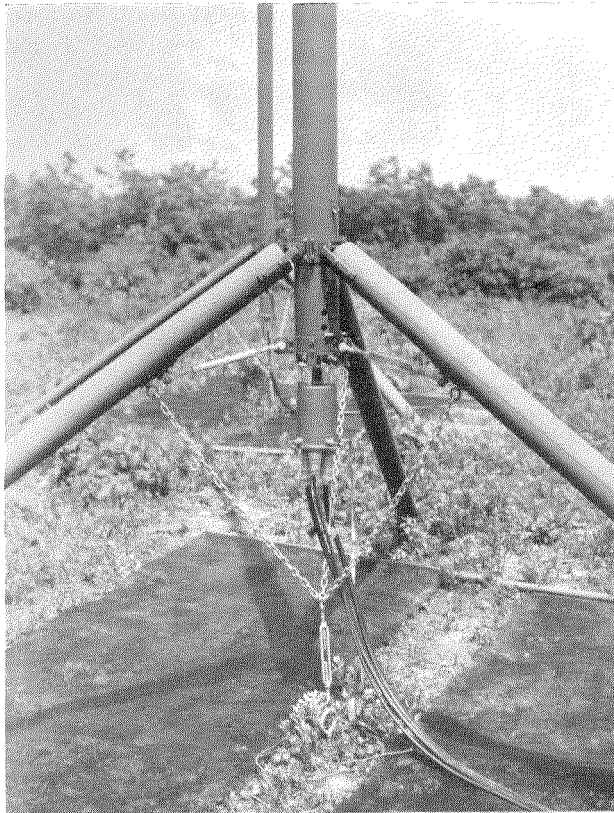
Fig. 3—The connections to the base of the center antenna of the wave-collector system may be seen above. Two flexible solid-dielectric lines are used.
