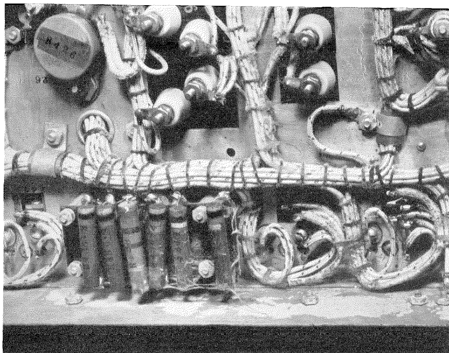
Under side of chassis of indicator box after tropical service. Fungi on insulating material lower insulation resistance and structurally destroy the material. Note corrosion on metal chassis.
